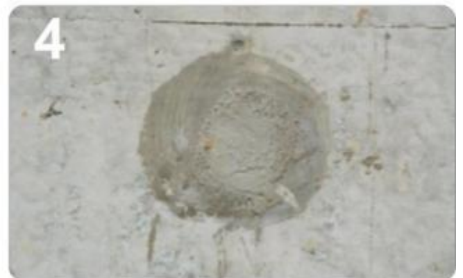
4 Patch the "hole" by cement + latex Trám lỗ ty bằng vữa + phụ gia latex
