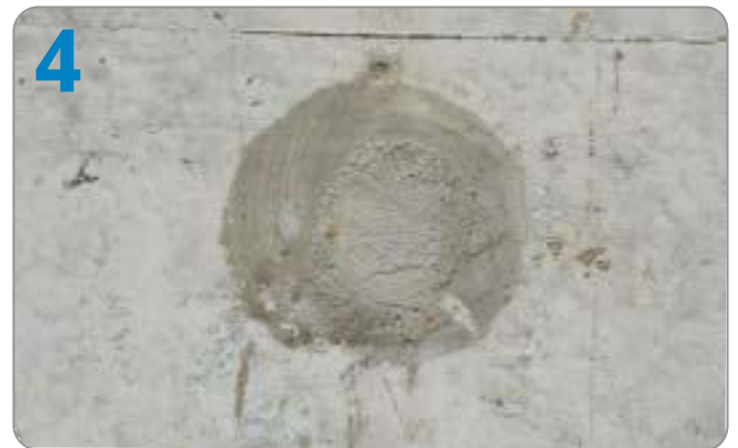
PATCH THE "HOLE" BY CEMENT + LATEX TRÁM LỖ TY BẰNG VỮA + PHỤ GIA LATEX
